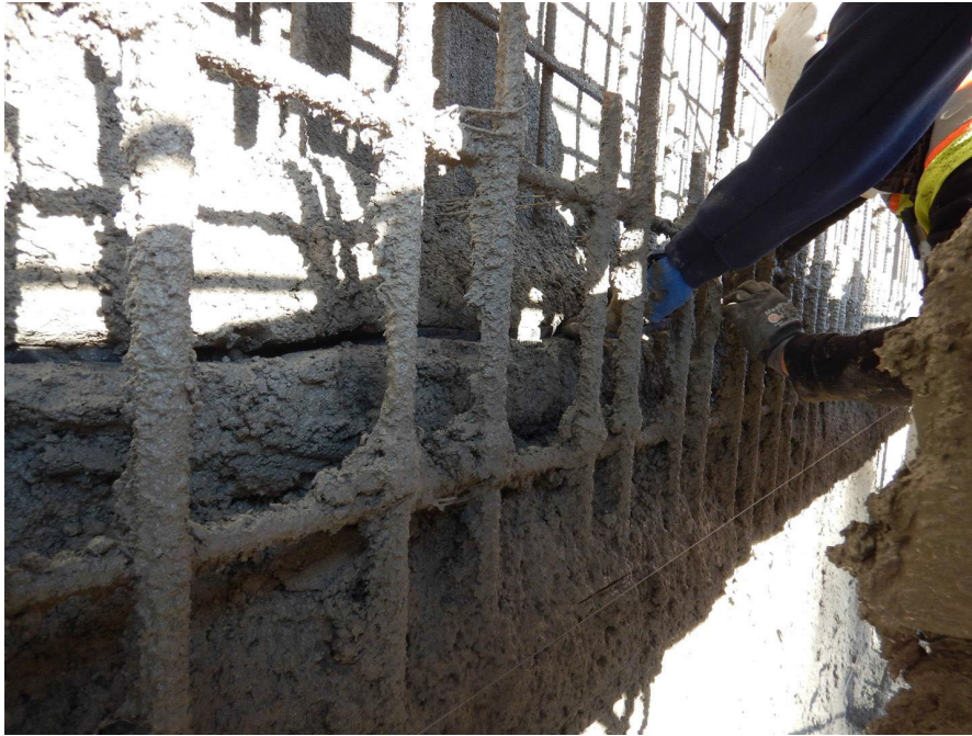
PHOTO 1: SHOTCRETE LIFT JOINT
